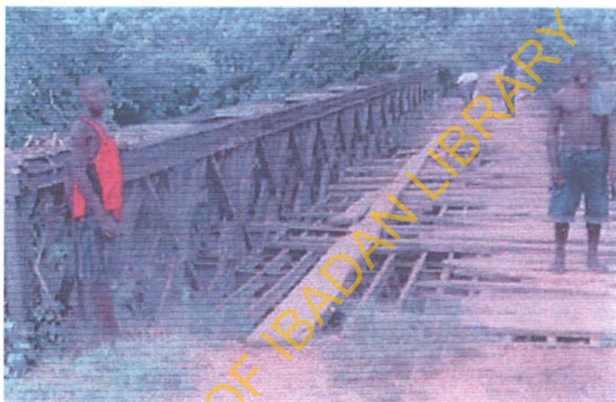
Plate 6: Dilapidated bridge linking the conservation area with Uyehe Community
