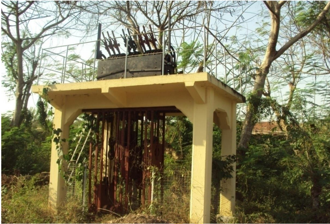
Plate 4.3: Signal Control Point at Erunmu Station, Ibadan.
