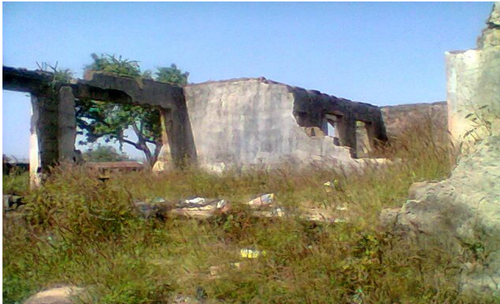
Damaged building at Jos Jarawa
