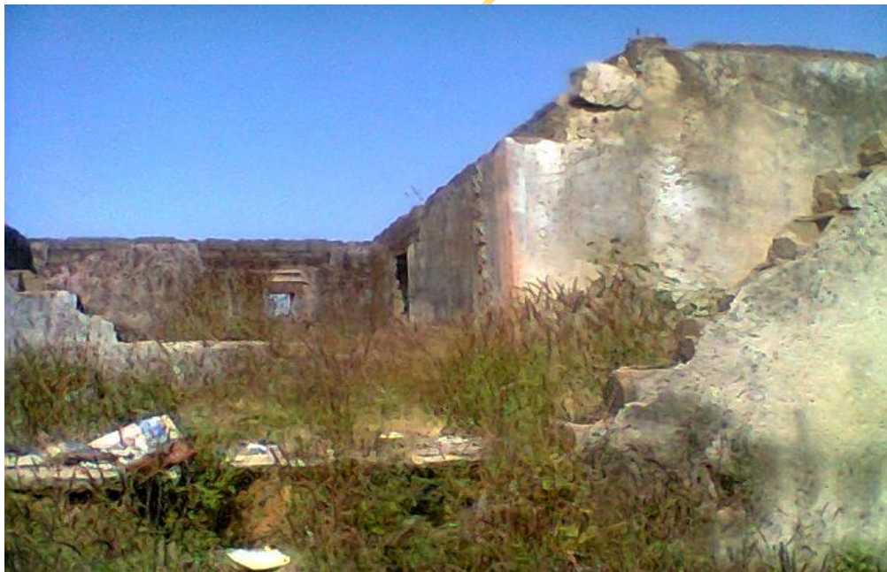
Damaged building at Jos Jarawa
