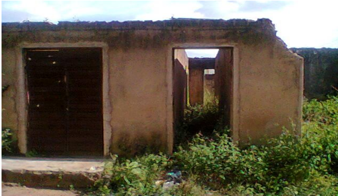
Damaged building at Rwang Pam, Angwan Doki
