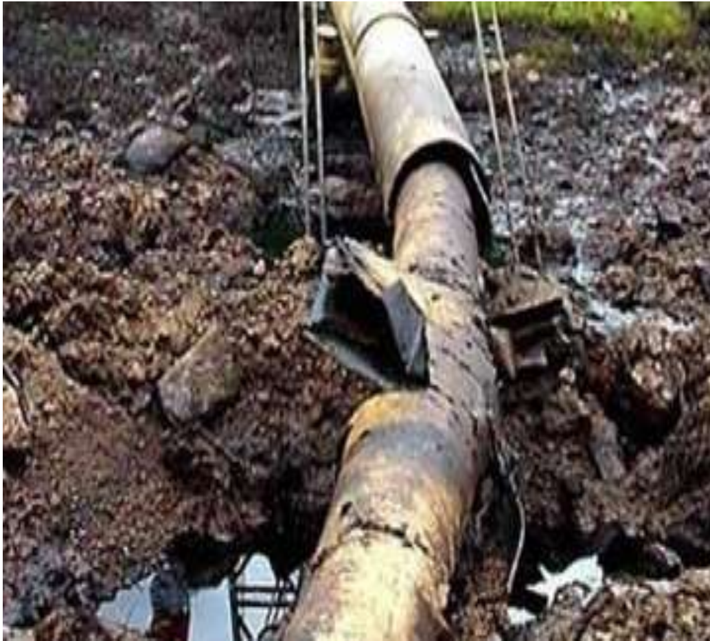
Fig. 1.10: Picture showing vandalized pipeline at Baruwa
