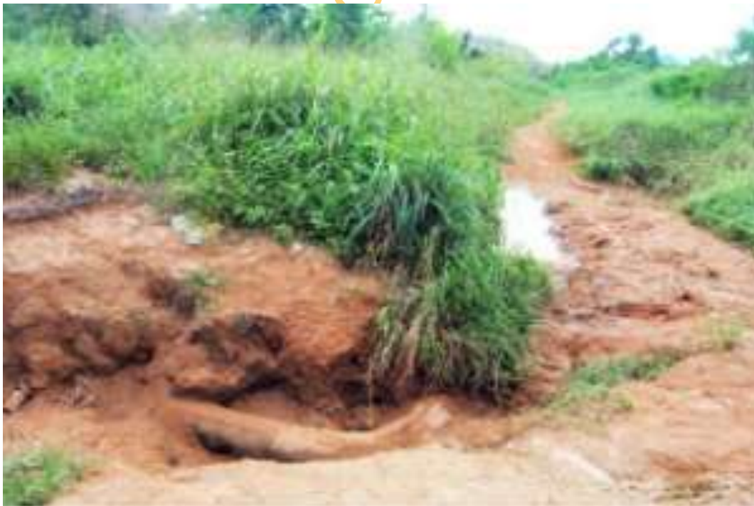
Fig. 1.11: Picture showing exposed vandalized pipeline at Baruwa
