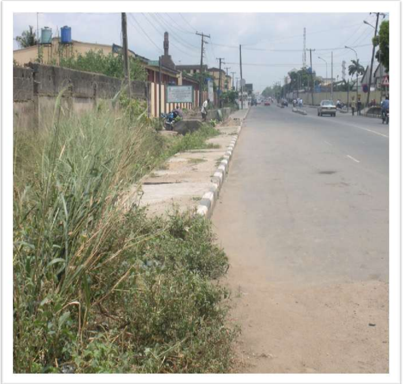
Plate 4.5: Walkway with Grown Weeds along WEMPCO Road.
