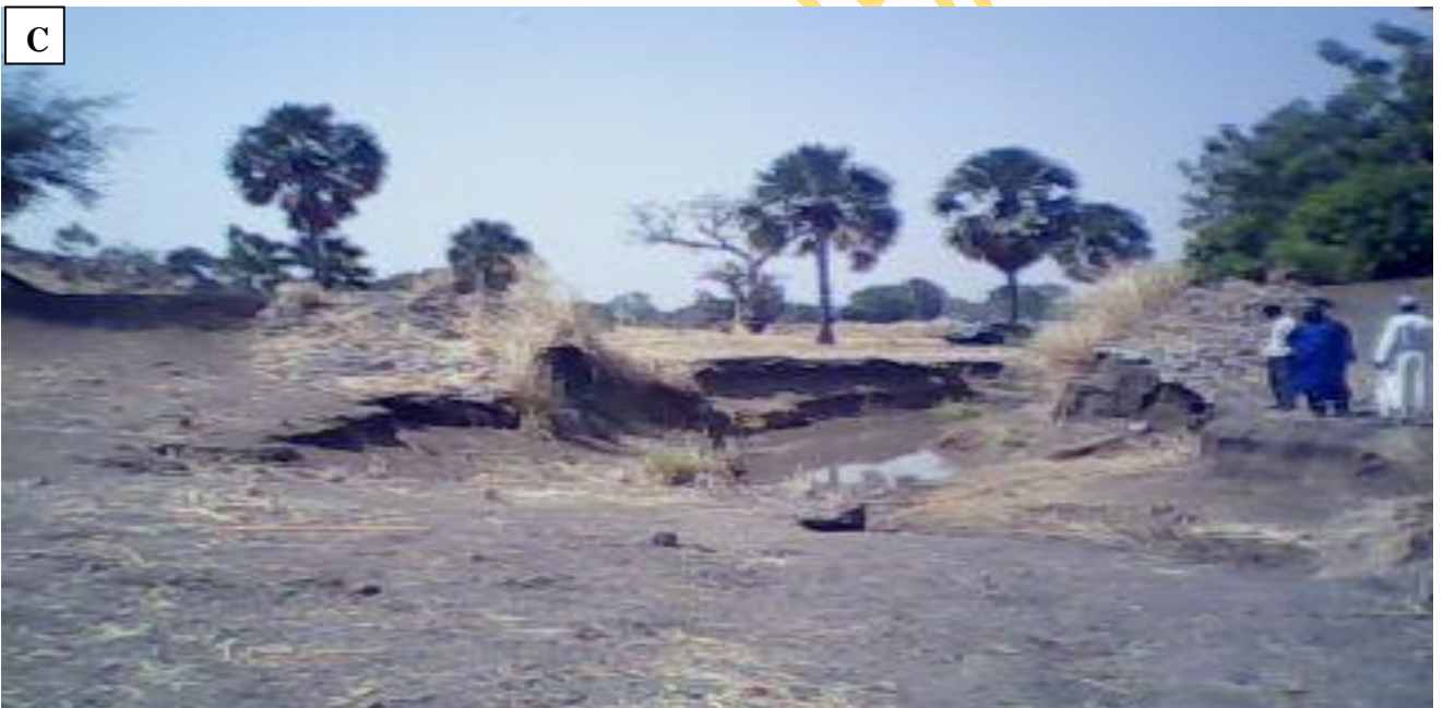
Fig 4.22; Nzuzu dam failure
