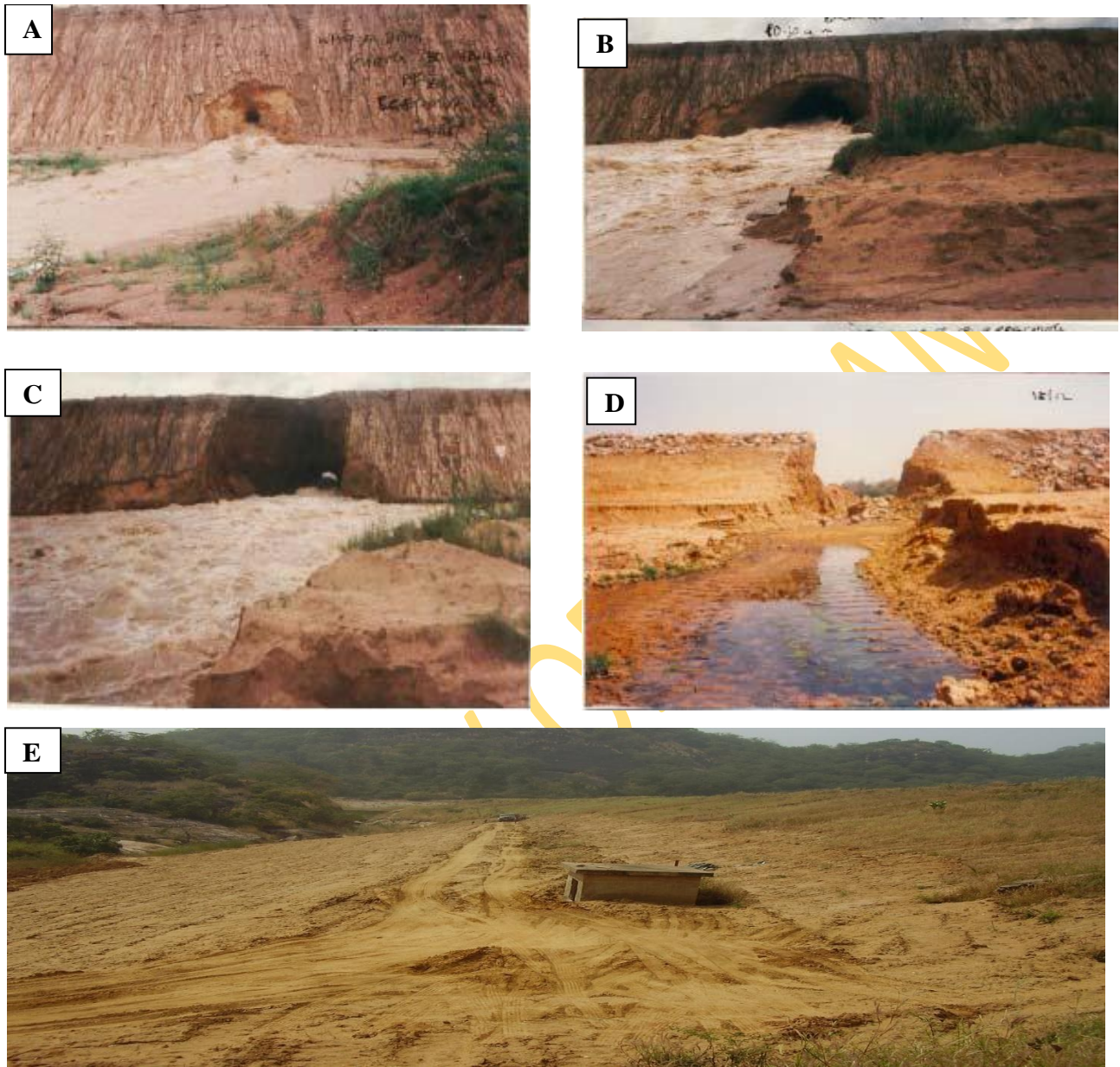
Fig 4.23; Waya Dam Failure (Seepage and piping failure) (source: Bada, 2008)
