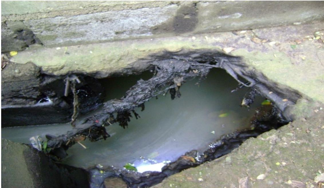
Appendix 2: Effluent channel of Hoesch Pipe Mill Ltd in Ikeja Industrial Estate
