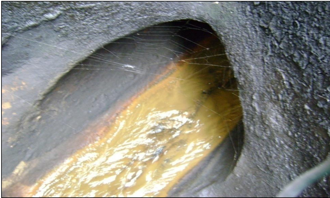
Appendix 4: Effluent channel at the central treatment plant receiving all effluents in Ikeja Industrial Estate.
