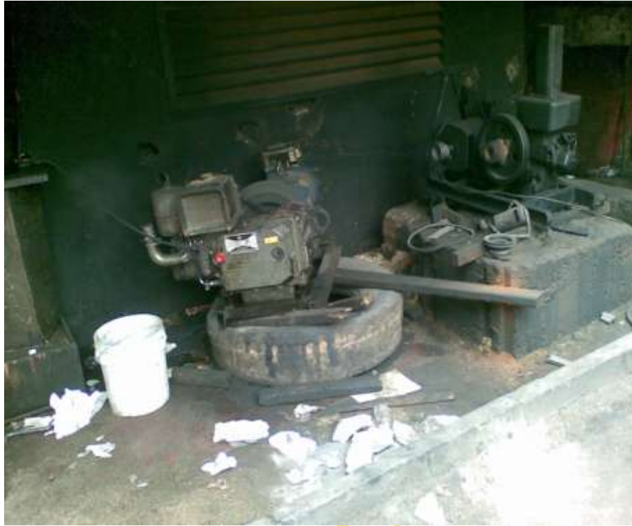
Plate 4.1: Poor conditions of Electric Generators
