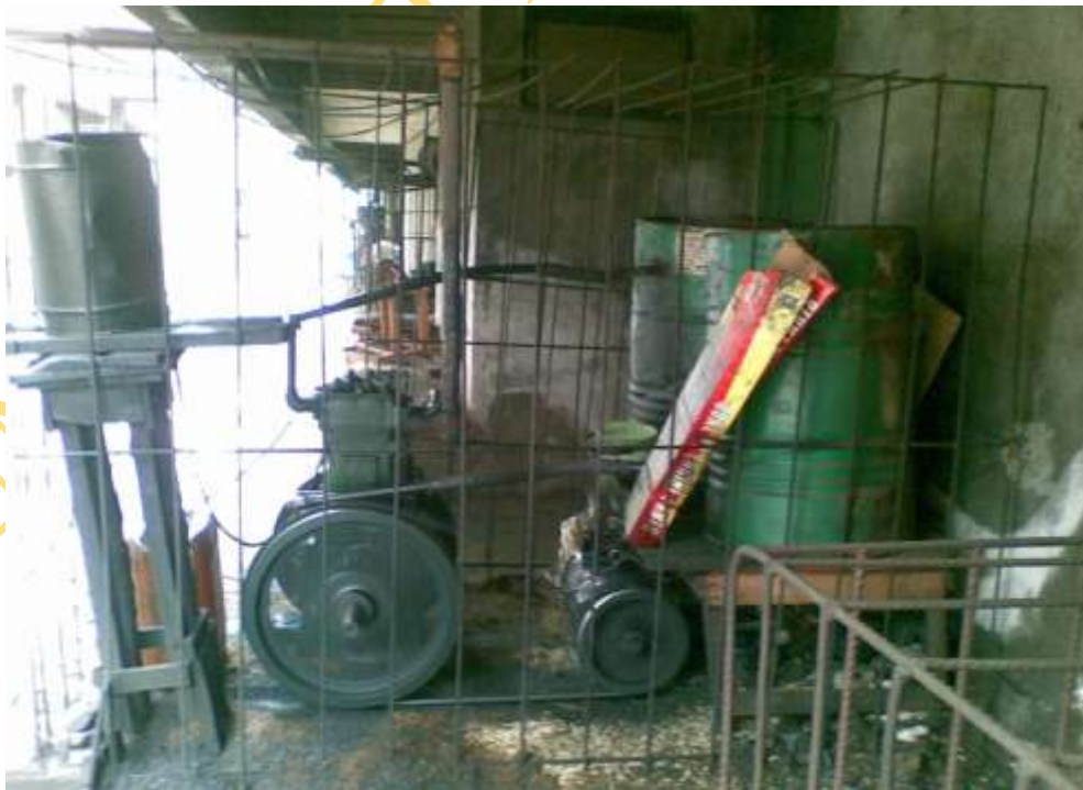
Plate 4.2: Exposed engine generators
