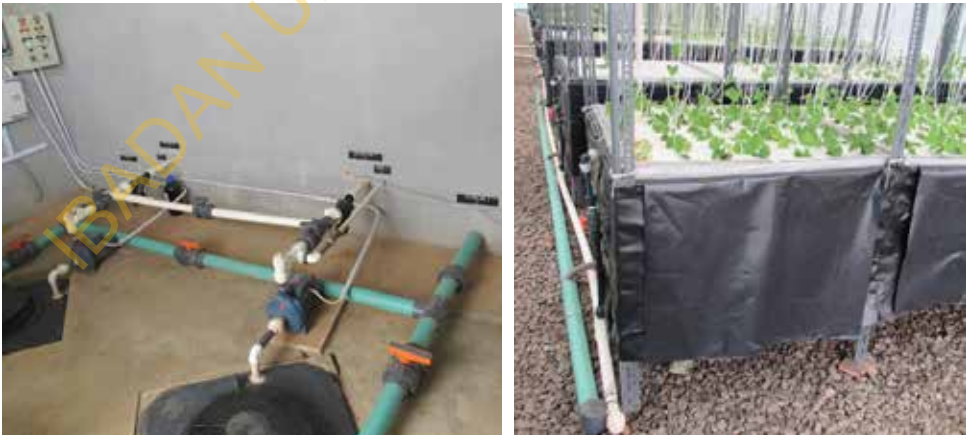
Figure 13. Piping in the power house (left) and pipes for feeding the plantlets in the boxes (right).
