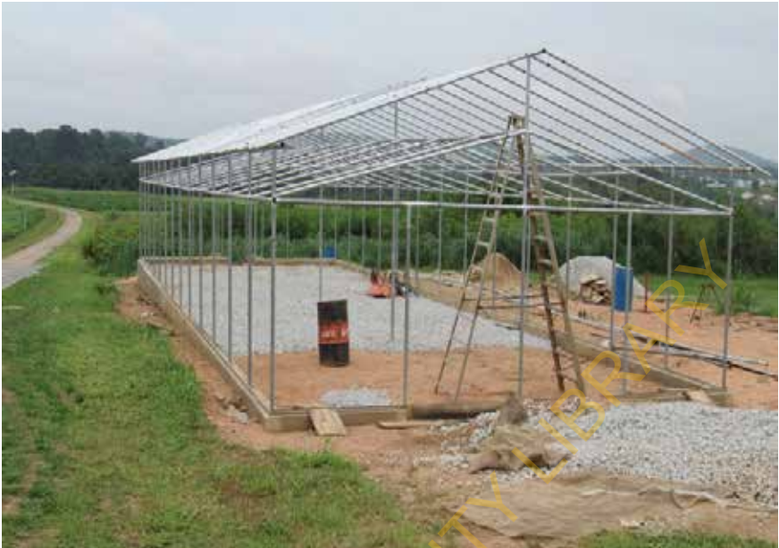
Figure 6. Full establishment of the solid structure for a double ceilings screen house type.
