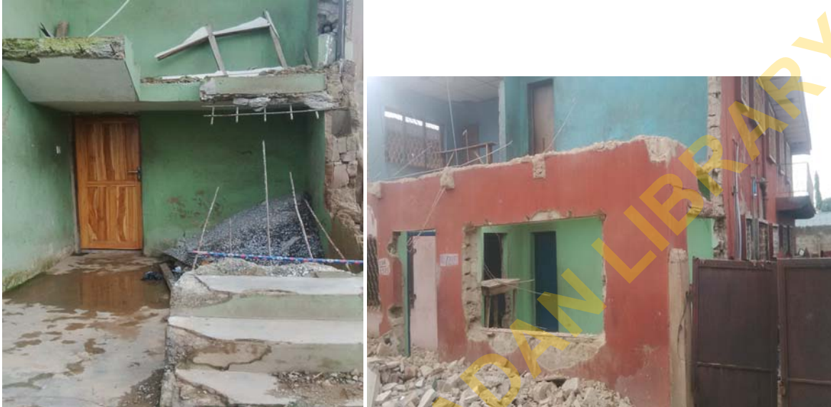
Plates 4 and 5. Showing the partial demolished state of cases 3 and 4
