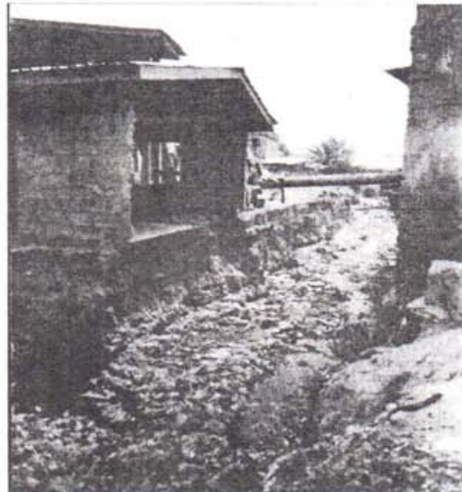
Plate 2: A Building under Threat along Water Channel at Alaro Area.
