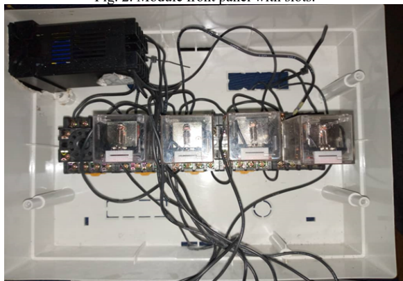
Fig. 4. Inner view of panel box while development was ongoing.
