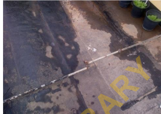
Plate 5: Broken water pipe.
