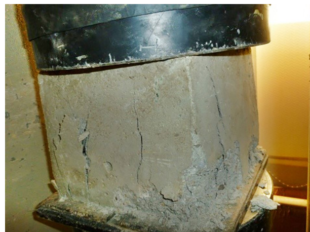
Fig. 1. Failure of cube (Photograph by Author)
