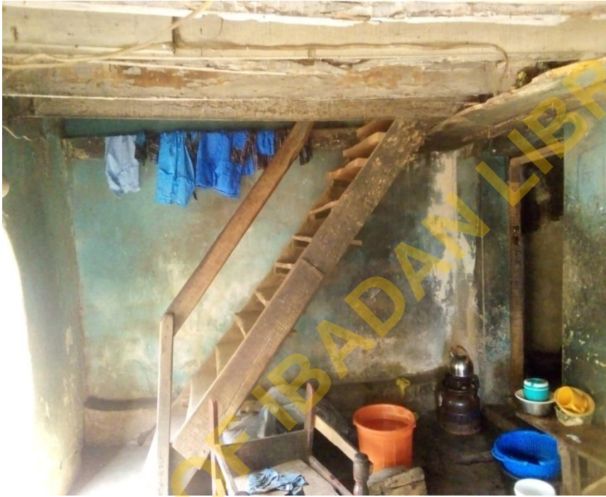
Figure 5.8: A non-habitable, dilapidated room, Bere. Source: Fieldwork 2022
